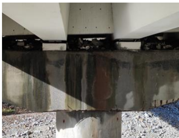
Figure 12. Bridge B: reinforcement oxidation.
