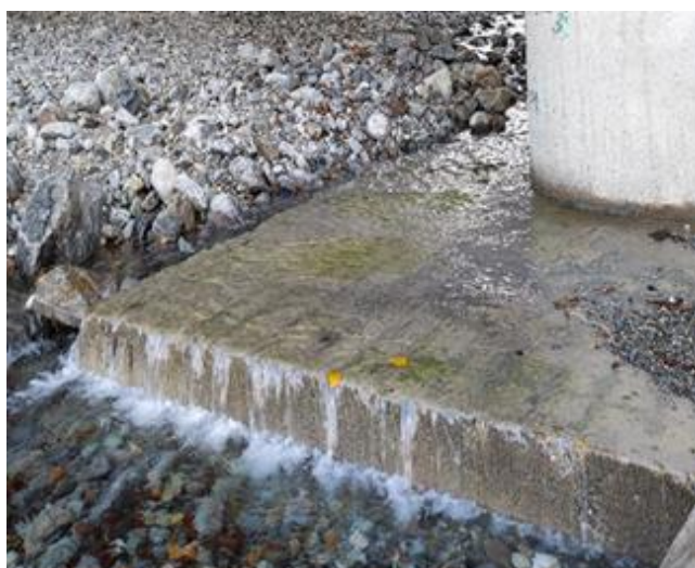
Figure 13. Bridge B: undermining of foundations.
