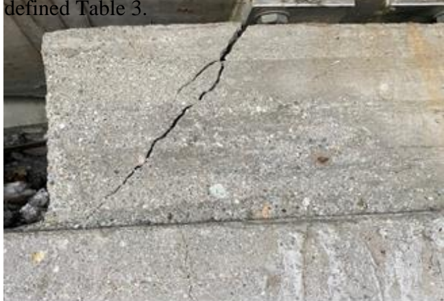
Figure 10. Bridge A: compression lesions on the central bearings of the abutments.
